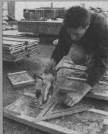
An employee with contractor George W. Davis works on Arista Place, a Watsonville development that includes 14 single-family homes.
